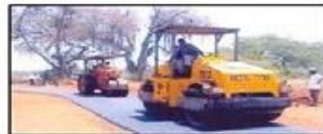
The mix known as waste plastic-aggregate bitumen mix can be used for road laying at 110-120°
